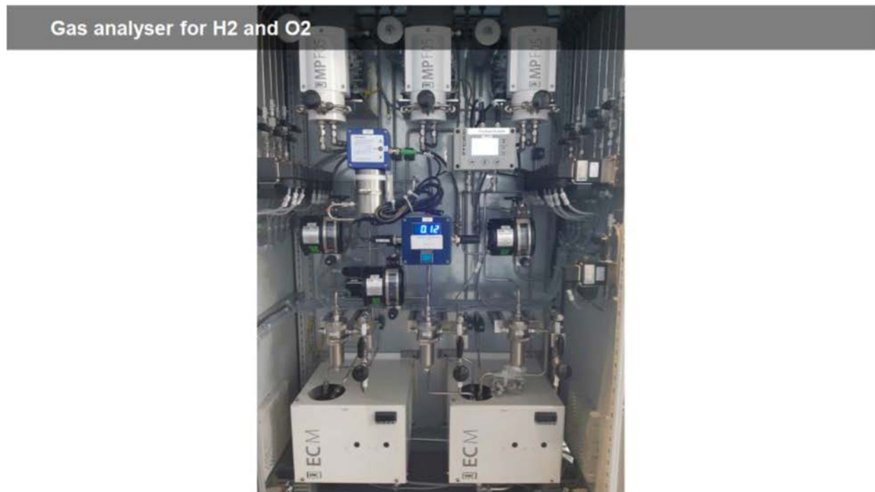
Gas Managment Plant.
